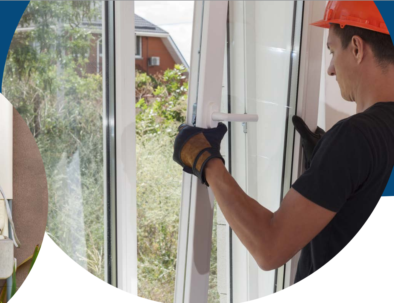
Heat Pump and Energy Efficient Windows
